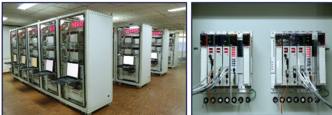
Figure 14. Nucon 1000 programmable logic controller from ECIL.
